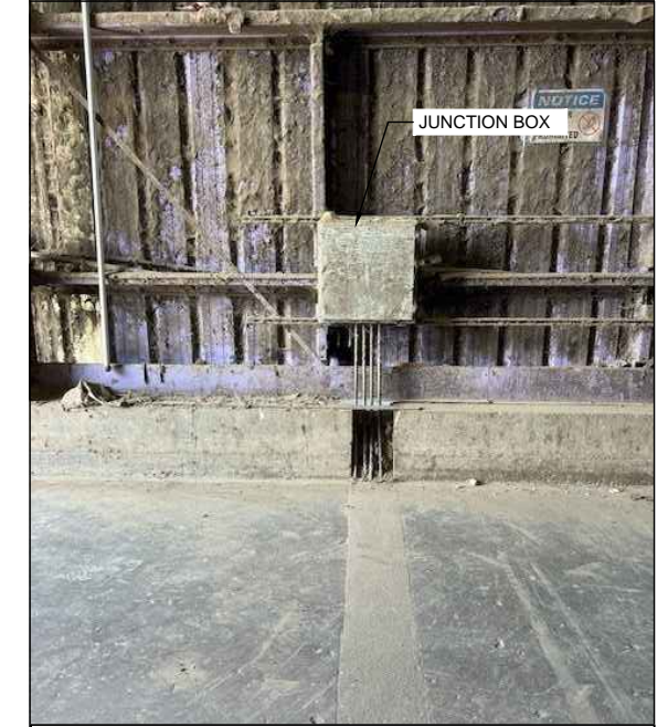
D - JUNCTION BOX LOCATED ON - WEST WALL
